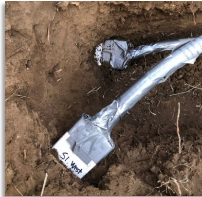
Figure 44. Soil moisture sensors inserted horizontally into a trench face, 15 and 30 cm below the soil surface. Note the horizontal offset between sensors to reduce mutual interference. Sensor cables have been fed through flexible electrical conduit for protection from animals. The tape is wrapped so that no portion of the sensor cable is exposed. Photo: Joel Biederman
