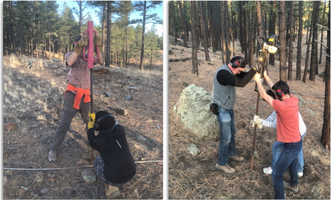
Figure 33. Driving T-posts into rocky soils near Flagstaff, AZ. Post location and rotation are first set with a manual post pounder, then a second team drives the post to the desired depth with a gas-powered driver. Photo: Joel Biederman.
