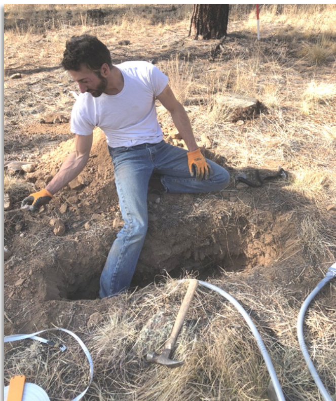
Figure 42. Adam Belmonte, Northern Arizona University, installing soil moisture sensors that have been fed into flexible conduit and sealed with heavy duty duct tape at Ft. Valley, AZ. Photo: Joel Biederman.
