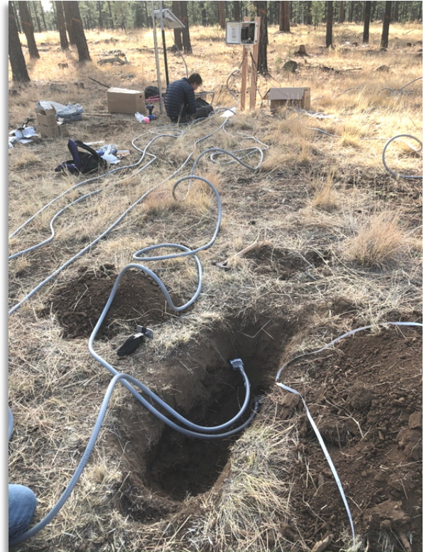
Figure 41. Snowtography station soil moisture monitoring system installation in progress at Ft. Valley, AZ. Solar panel and data logger are visible in the background, and soil moisture sensors, cables, and trenches are visible in the foreground. Photo: Joel Biederman.
